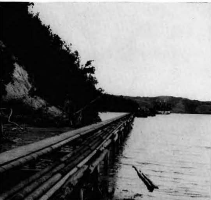
Oil and fuel lines on a jetty.
