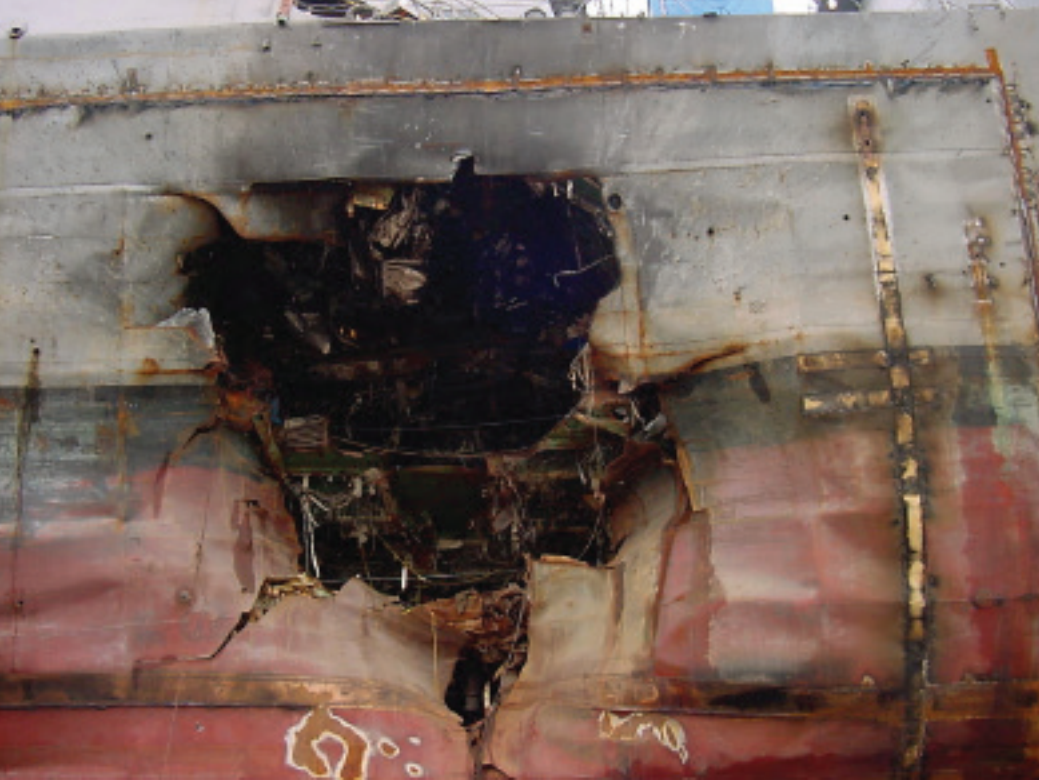
USS Cole 's damaged hull is shown clearly in this closeup. (Courtesy of James Parlier)
