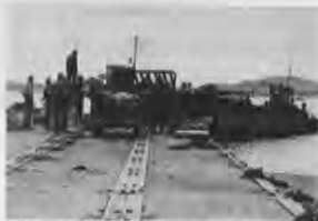
LCM pulls into pontoon pier at Walmi Do Island, Korea, to unload supplies.
