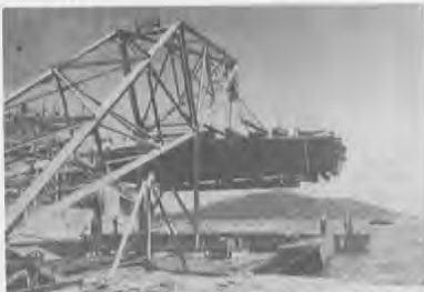
The 75-ton crane can lift a P.T. boat out of the water.
