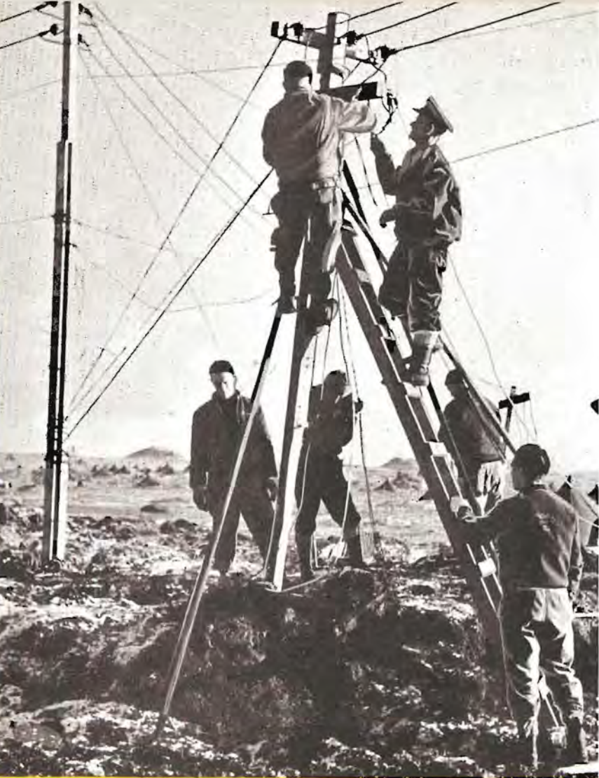
● One of the principal jobs of the Seabees is the installation and repair of power and light facilities at advance bases. This picture was taken at Amchitka.
