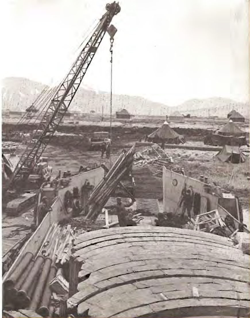
● Alaskan Sector. Seabees are unloading lumber from an LCT with the aid of a crane. The curved sections in the foreground are parts of Pacific huts.
