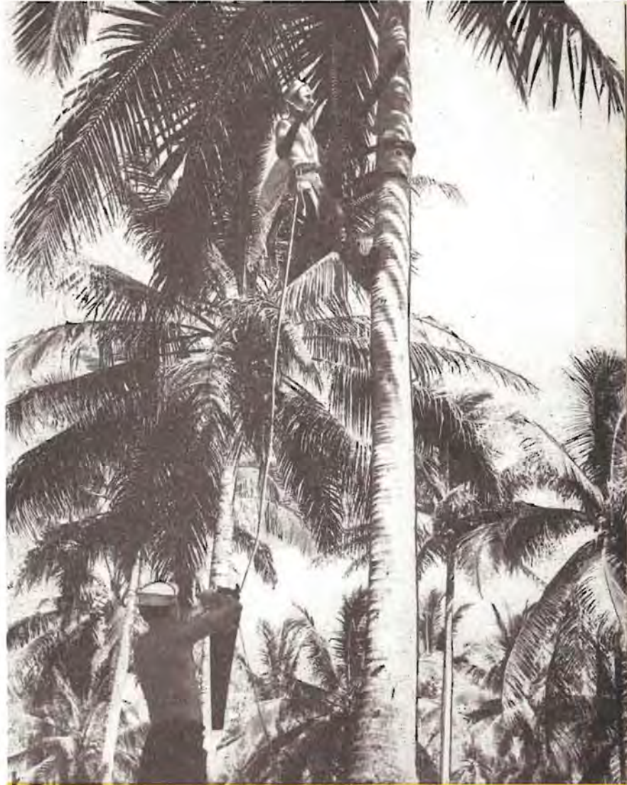
● At the Naval Base on Espiritu Santo, Seabee electricians rig support arms on coconut palms for a power line. The tall straight palm trees are perfect for this purpose.
