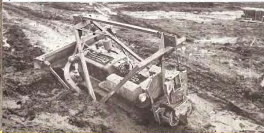
● One of the difficulties encountered by Seabees building roads on Kiska is the deep mud, while at other points on the same island volcanic rock had to be blasted to clear the way.
