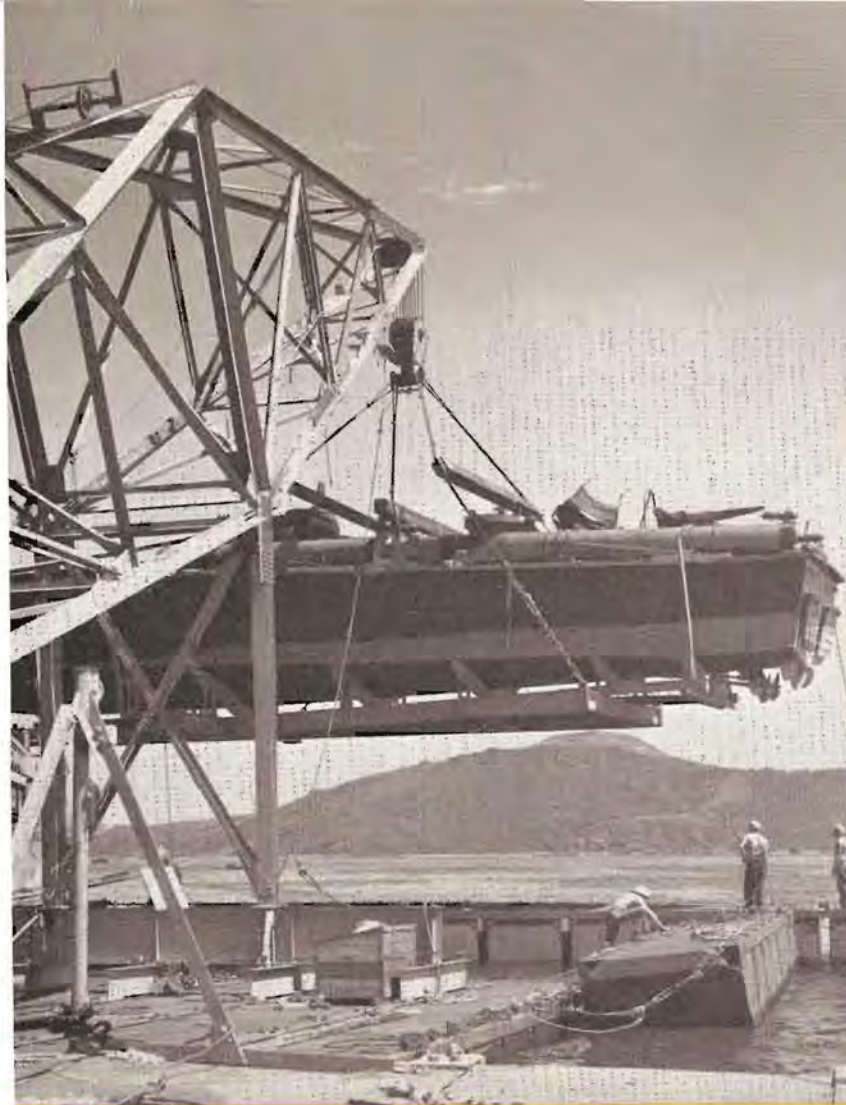
● A seventy-five ton crane on a pontoon barge lifts a P T Boat from another pontoon barge moored alongside. The scene of this photograph is at a Mid-Pacific Island base.
