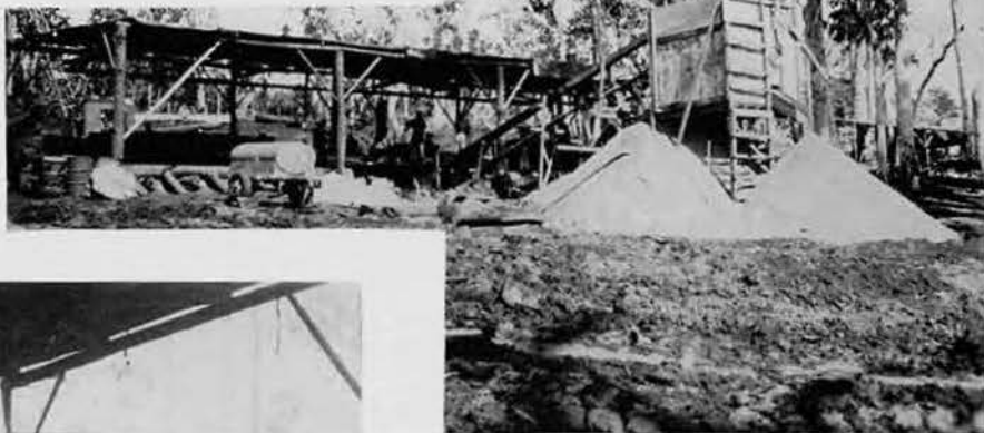
This Philippine sawmill turned out over a million board-feet of fine hardwood boards in less than three months . . .
