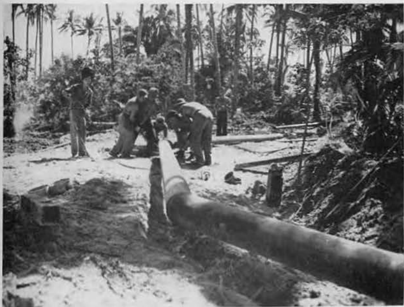
Fresh water line in the Philippines
