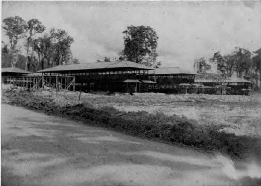
- These 100 men barracks were designed and built by the 91st for a naval receiving station in New Guinea
