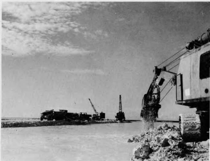
Excavating coral with a drag-line and rushed up to the rollers and graders on the Strip.
