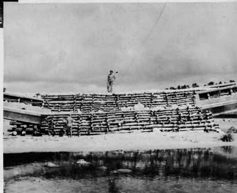
(Right) The same bridge shored up and re-vamped . . . ready for use, pending the possibility of Jap sabotage during the night to blow it up.
