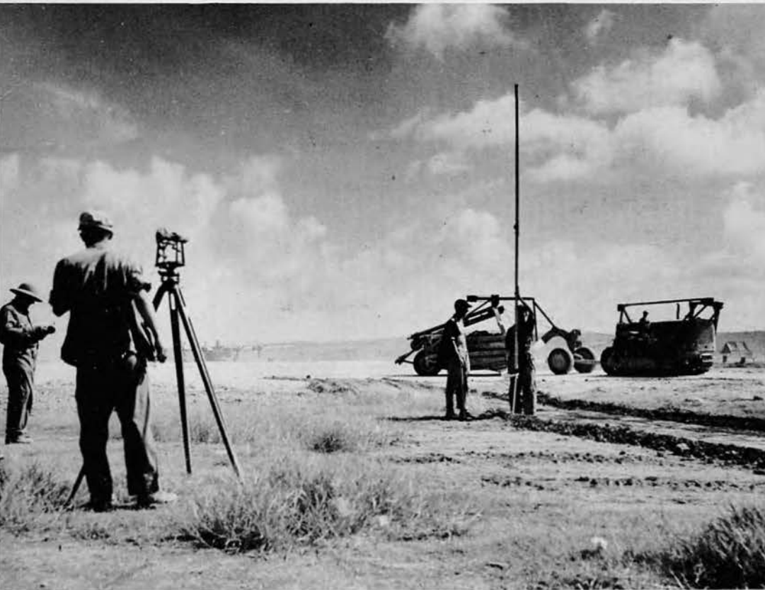
(Left) Preliminary survey for new East runway at Yontan Air Field. This was to be a "sister" bomber strip to the adjoining field.
