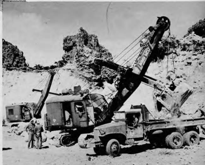
The big 6, our largest shovel gouges out coral after the blast and loads it into waiting trucks.
