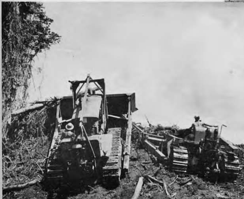
Expert handling of the "Iron Broncos" while building revetments around parking areas of bombers.
