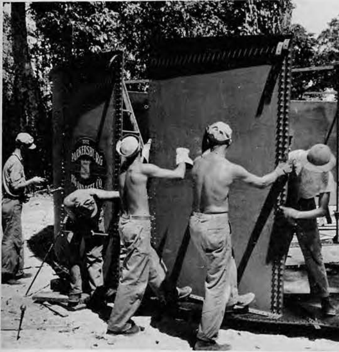
Octane Gas tanks erected inland, supplied fuel to the air-field.
