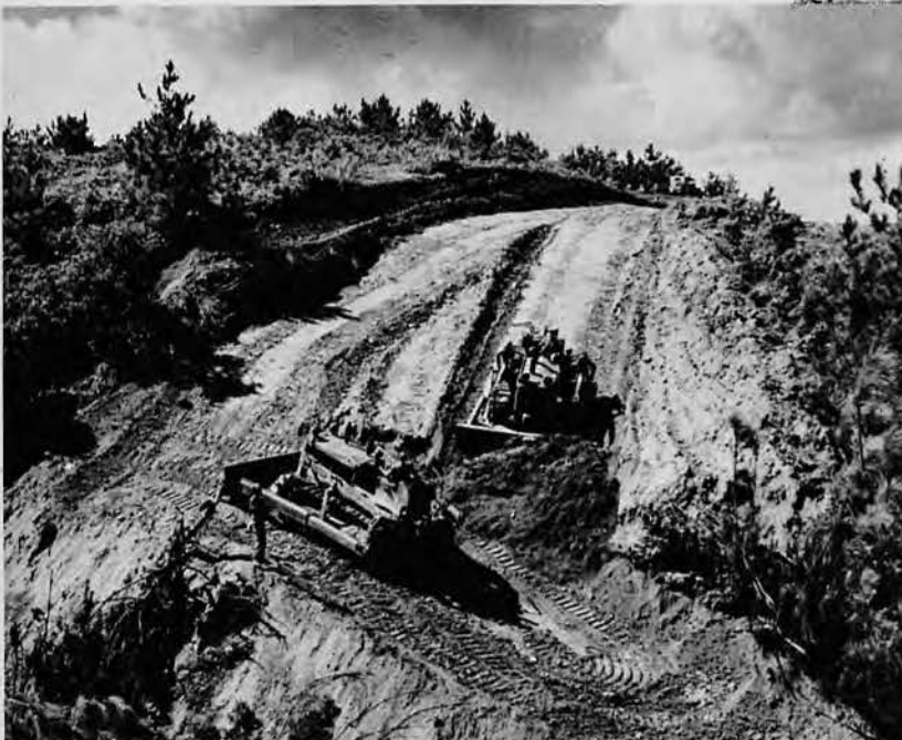
(Left) Two bulldozers spreading the earth as men, machines, time and materials transform these acres of valleys into modern lanes for fast moving traffic.
