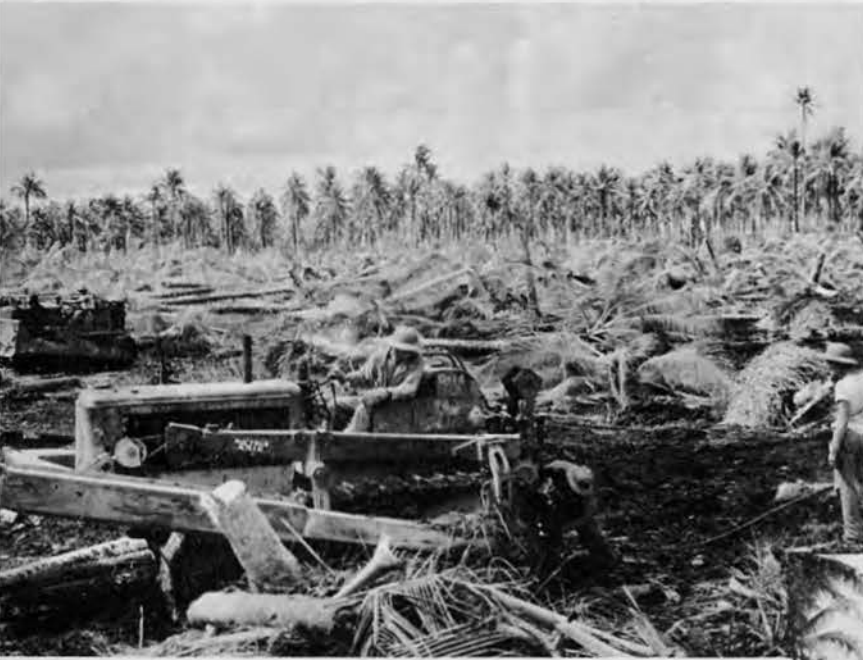
Logs are "snaked" to a nearby stock pile to be used later for general construction work.
