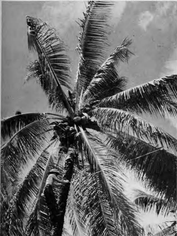
Telephone linesmen walk to the tree-tops and string the communication wires . . . with deftness.
