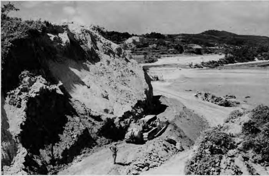
'Dozer cutting corners off a sharp curve. Eventually this ledge was levelled to meet the lower road, making it a two lane highway.
