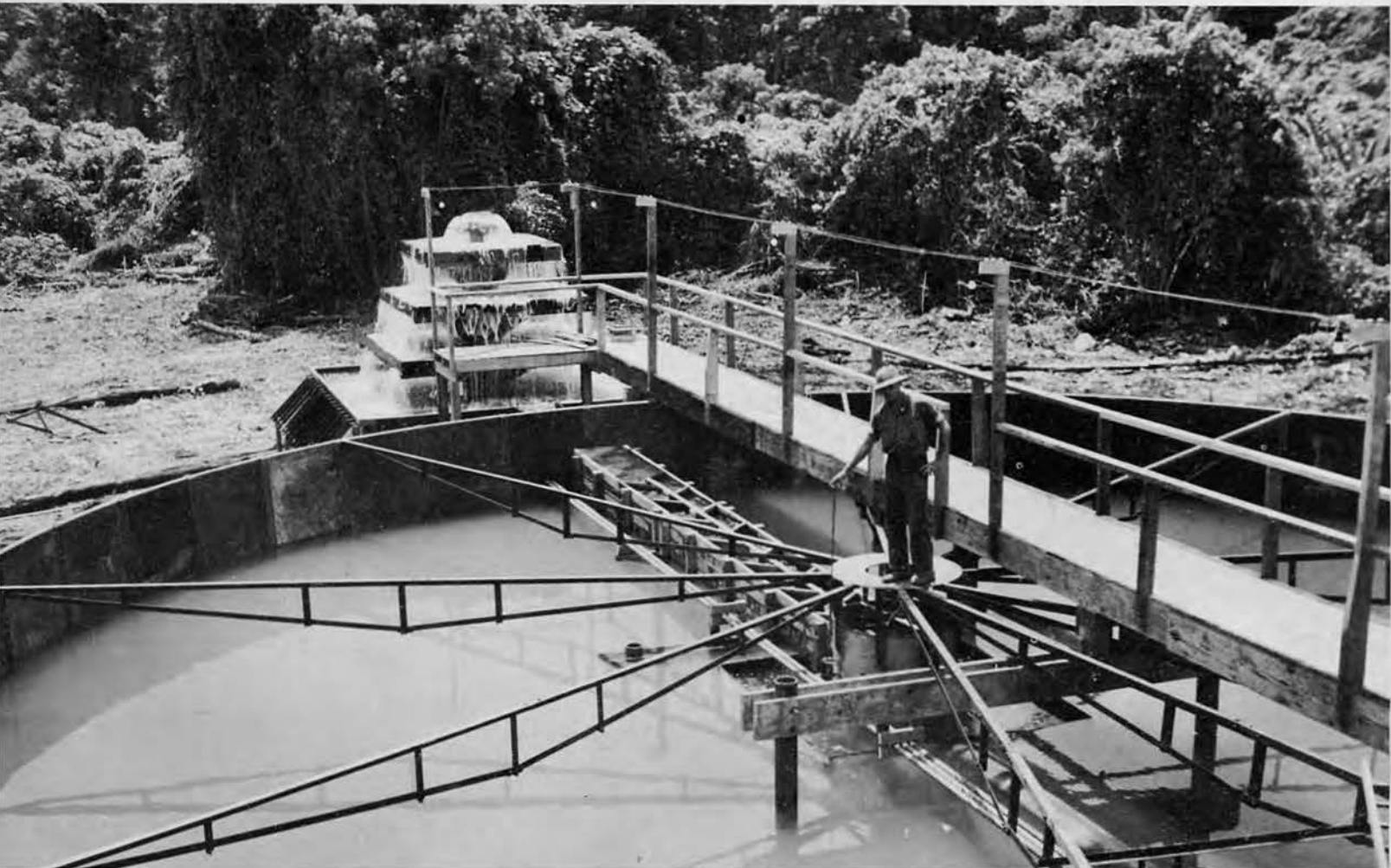
. . . where James C. McGowan, CWT, standing on steel trusses opens chemical controlling valve.
