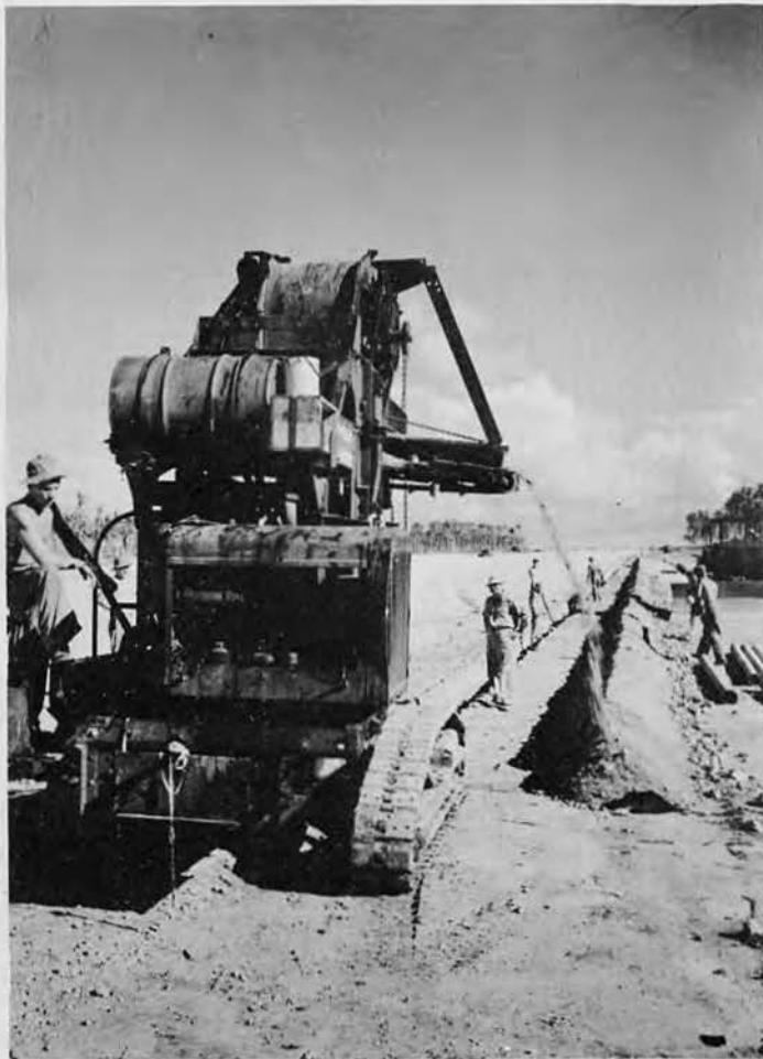
Ditch-digger cutting trench for the salt water sprinkling system to aid the compaction of the runway surface.
