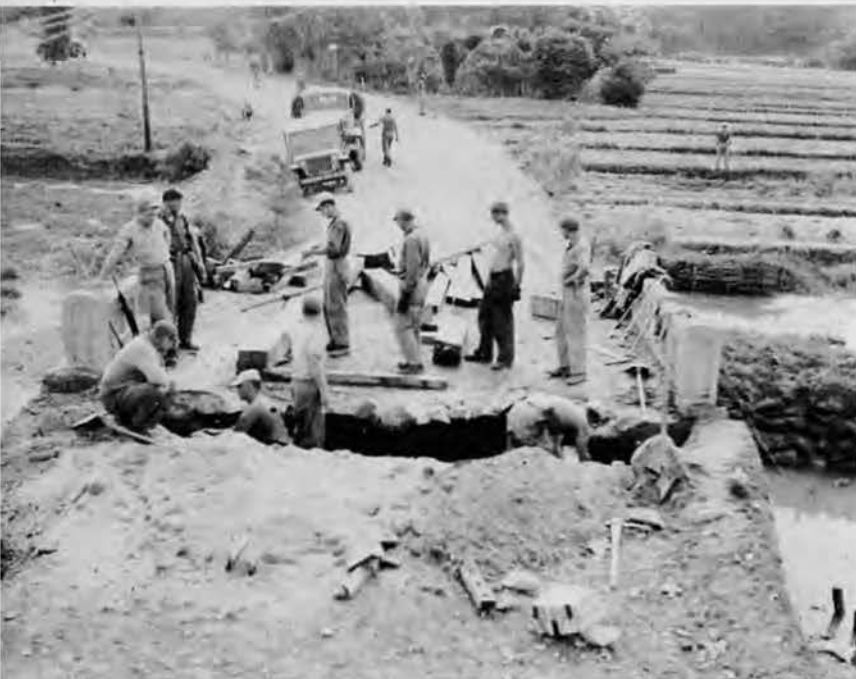
On a road subjected to sniper fire and treacherous sabotage, this bridge was constantly repaired after each sabotage incident.
