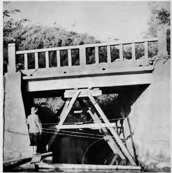
Inspecting "A" frame trusses which support bridge. This was the second repair job . . . sabotage had wrecked the first attempt.
