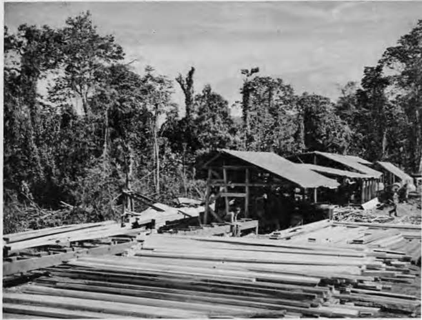
One of the most important building necessities, the Saw Mill, which broke "finished board" records.
