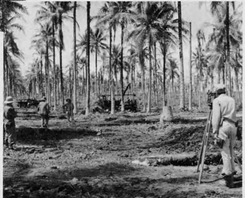
Neither rain . . . nor storms . . . nor the tropics kept surveyors or operators from their inevitable goal.
