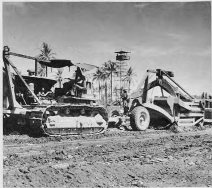
Upon completion of construction, the finishing touches are put on the shoulders of the field.
