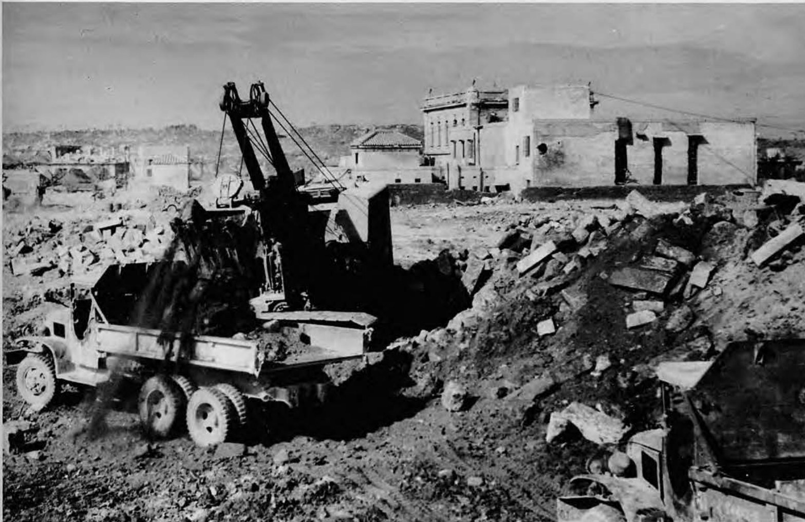
Debris from Naha City helps to build new roads. Our big shovel scoops up the famous city's remnants.
