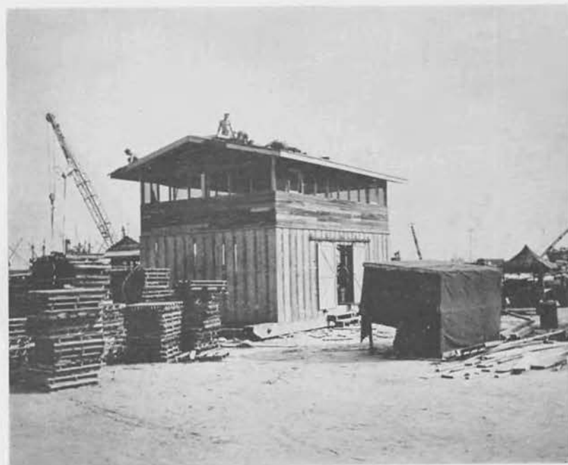
Gear locker for docks. Five such buildings were erected by the 53rd NCB.
