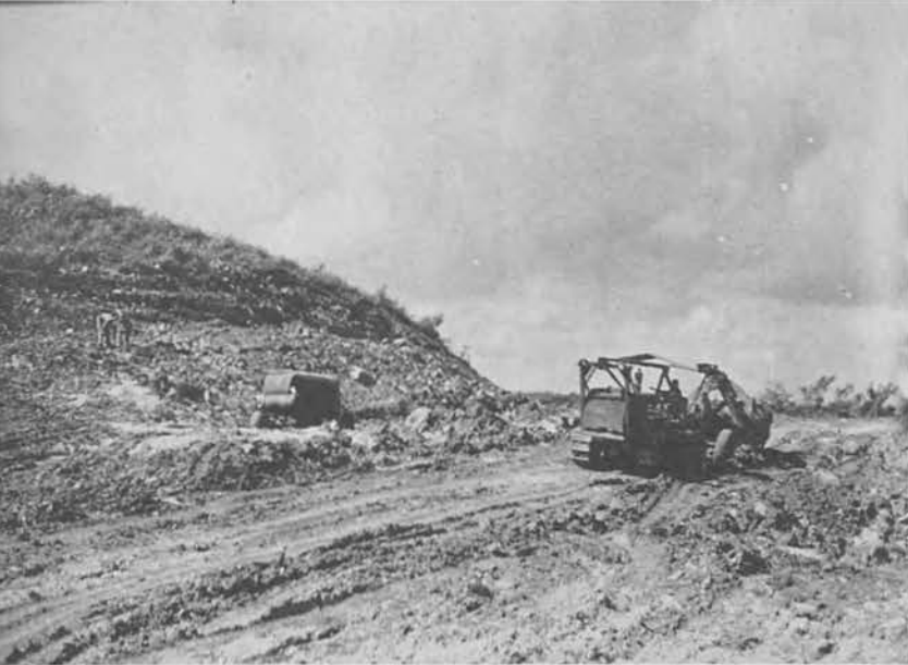
Initial grading operations on the Seawall Cut. Approximately 150,000 cu. yds. of excavation was removed.
