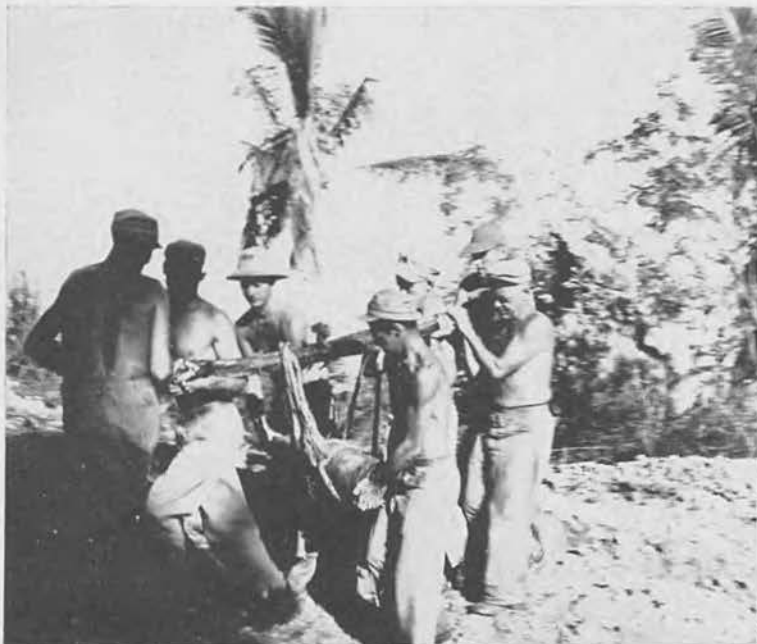
Demolition squad under Chief Winslow removing 8-inch Naval shell on Piti-Agana Road: Goss, Jay, McLean, Eidemiller, Bowden, Morris, Ch. Winslow.
