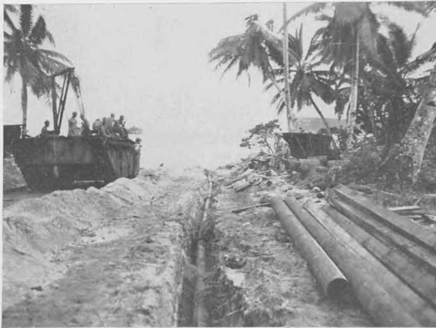
Installation of submarine pipe line from tank farm across reef to tanker discharge site. Approximately 1,500 lineal feet of pipe line lay on the reef.
