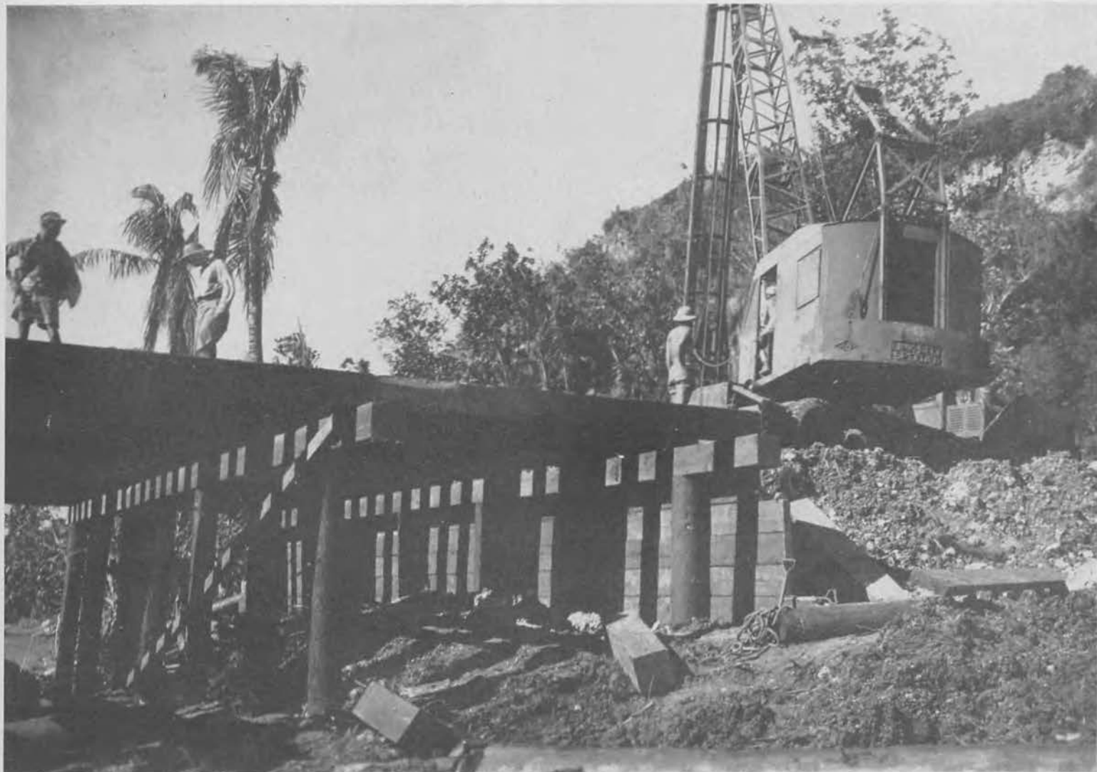
Scene on another bridge. Most structures are wood deck on wood piling bents.
