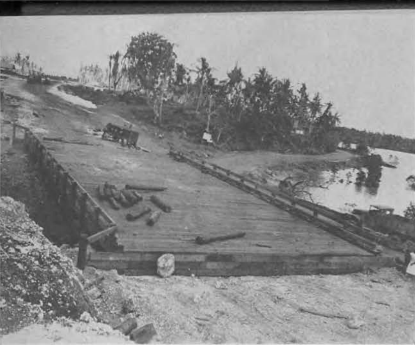
The first bridge constructed on the new road system of Guam, typical of several bridges built by the 53rd NCB.
