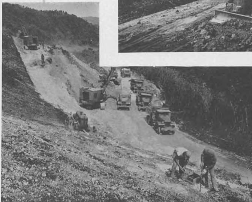
Above: Grading on the entrance road to the AROU Engine Test stands. Agat village is in the background.
