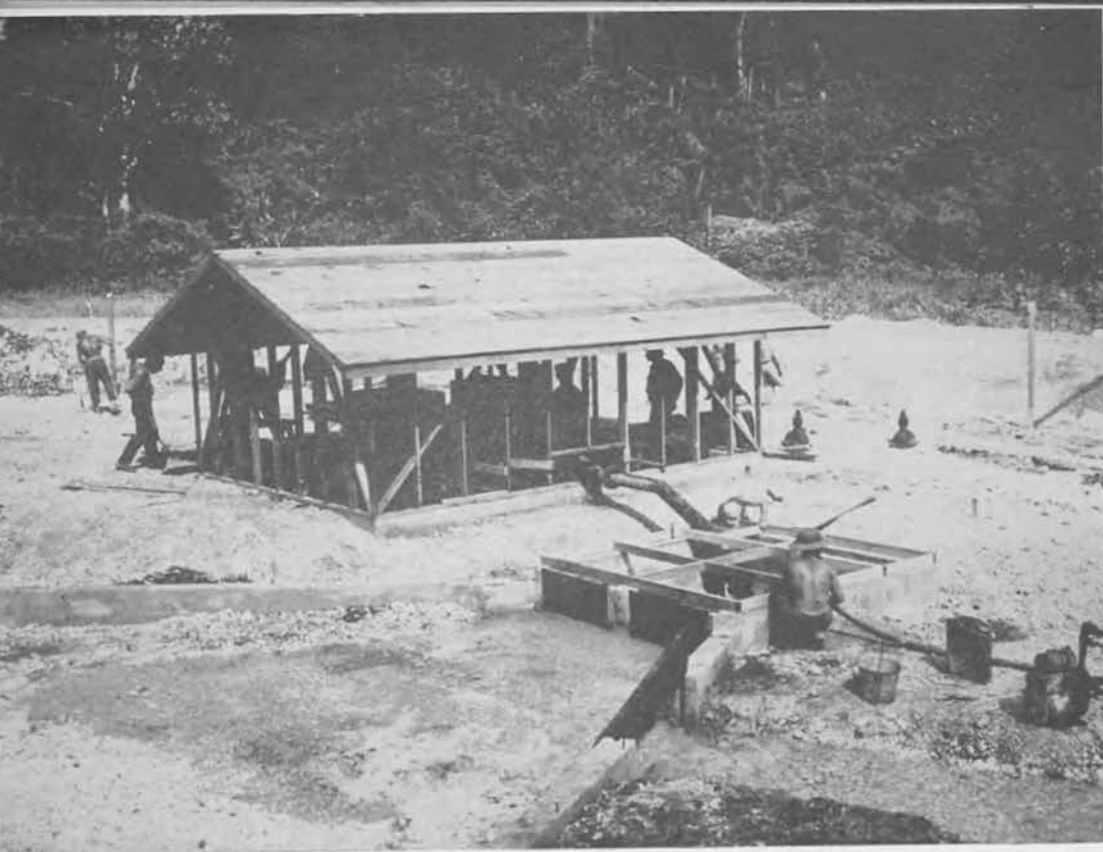
Bona Springs water development consisted of concrete pump and small pumping station. This project added about 500,000 gallons per day to the island supply.
