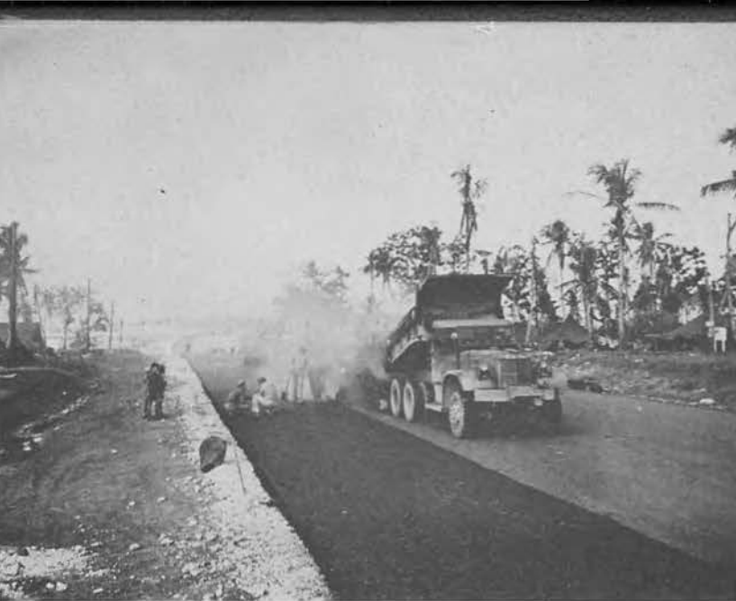
Paving near original site of 5th Field Depot on Marine Drive. Mid-December 1944.
