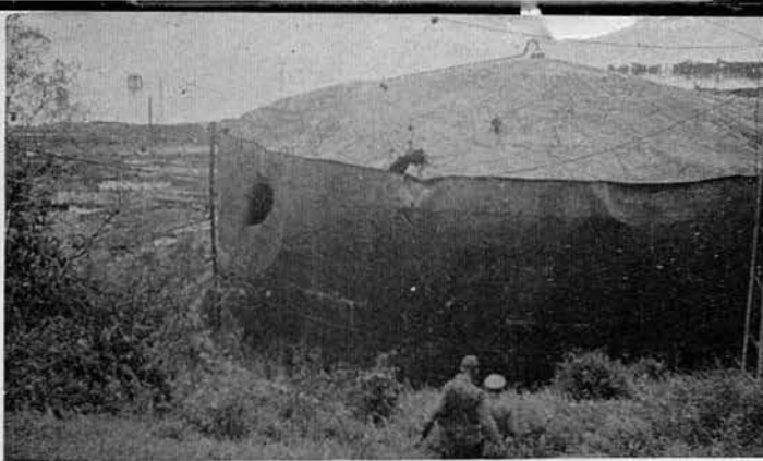
DAMAGED OIL STORAGE TANK
