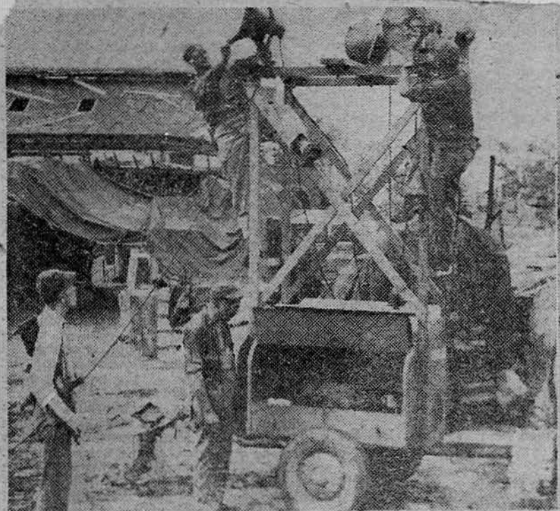
Fifth Seabees put up night lights for round-the-clock construction work to turn Balikpapan to full-fledged advance site in Far East.
