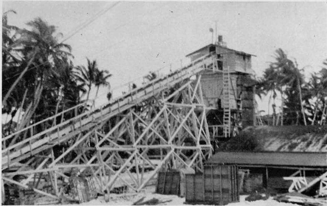
Concrete plant. Crusher plant out picture to left.
