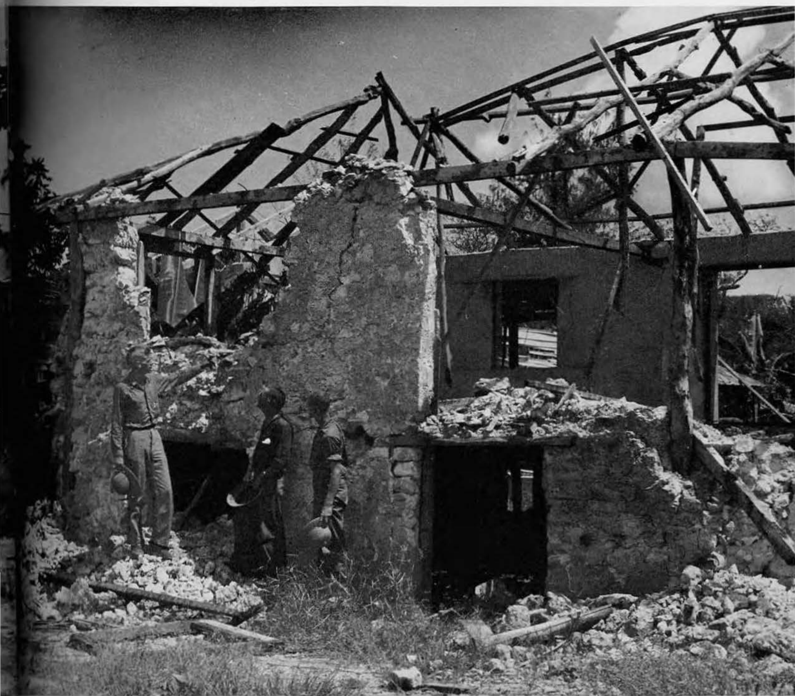
Stone walls reduced the fire hazard . . . but frame roofs offered no protection at all.
