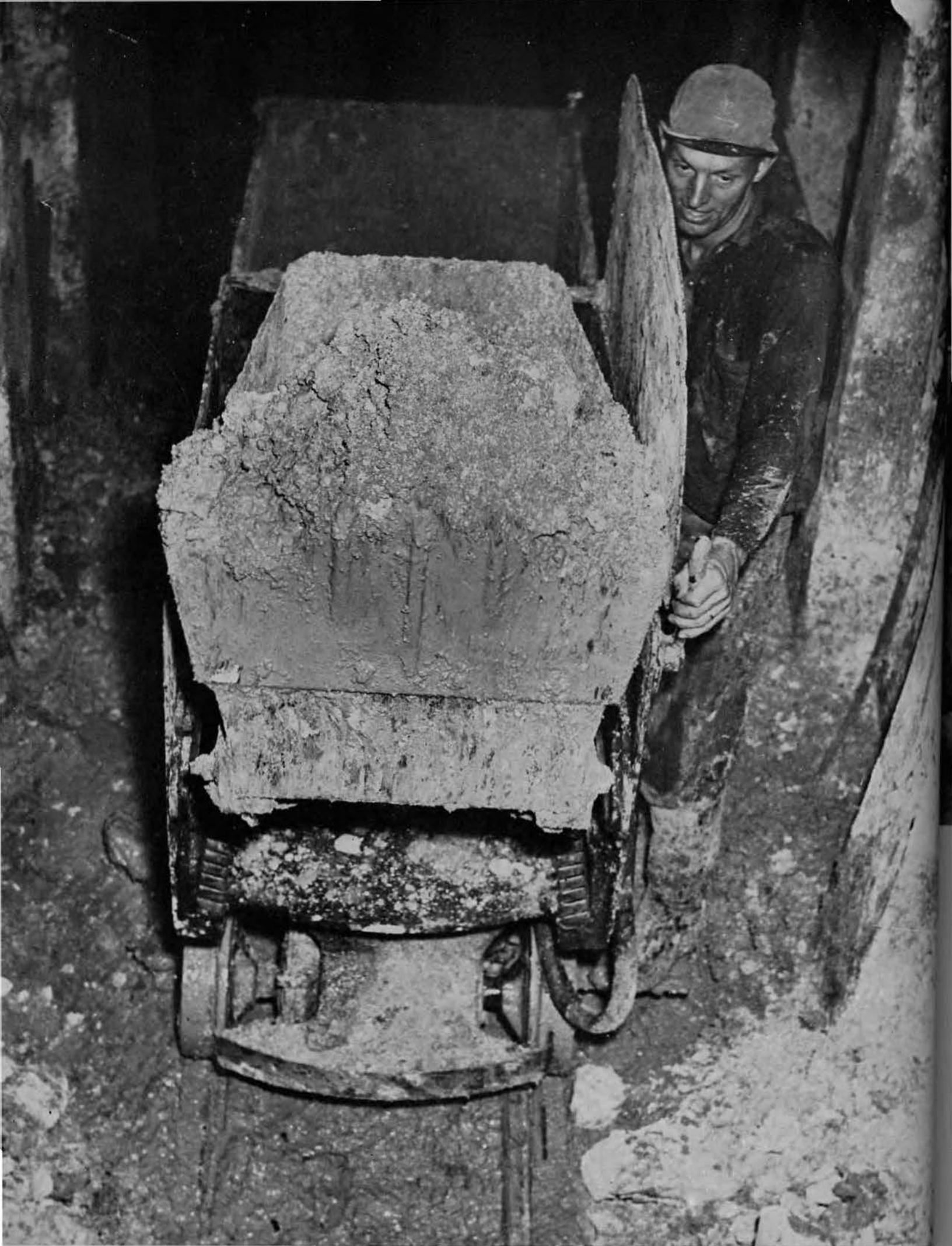
Alternate layers of hard coral and mud made progress on the job slow and dangerous.
