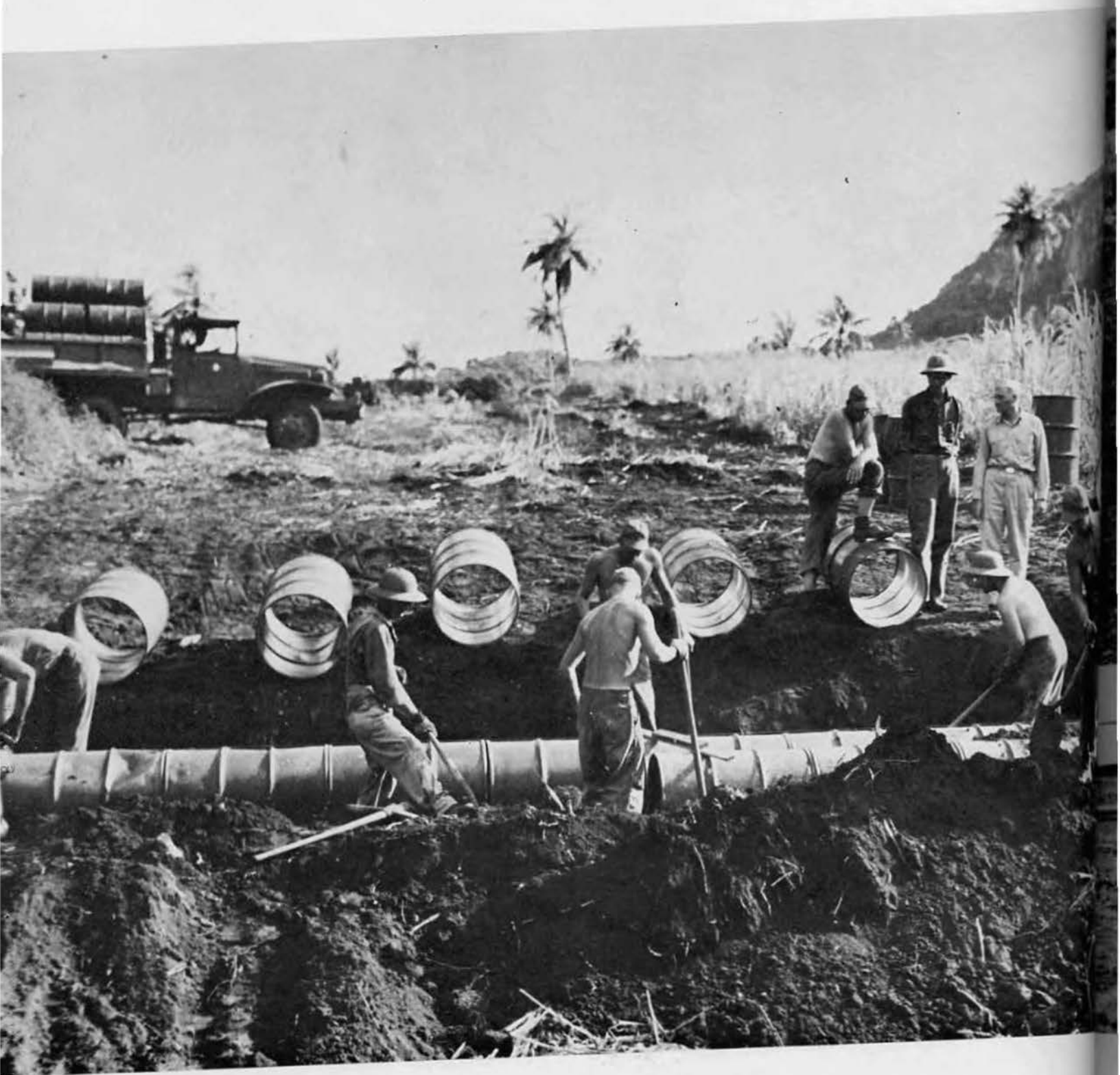
With a couple of short dry seasons wedged in between perpetual rains, special precautions had to be taken to drain the roads.
