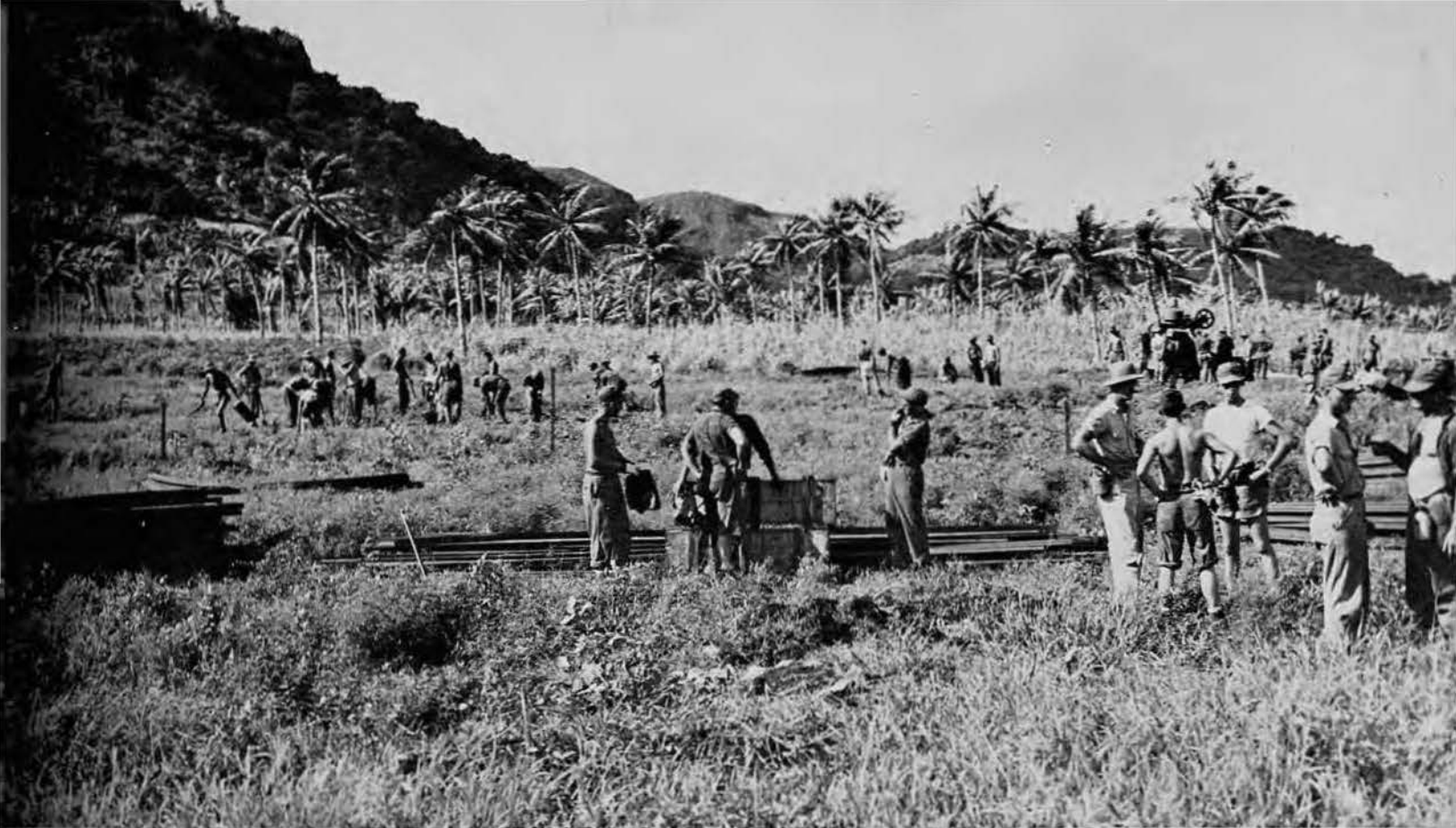
Every steel rib—every sheet of metal roofing had to be packed on our shoulders from the supply yard up the slippery, gooey hill to the building site.
