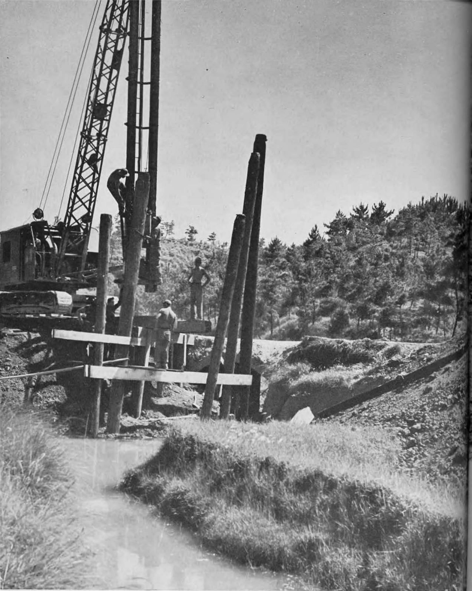
One of the major problems of road building was to lay road beds over seemingly bottomless rice paddies. The "salty" dock building crew sometimes had to move inland to give a hand.
