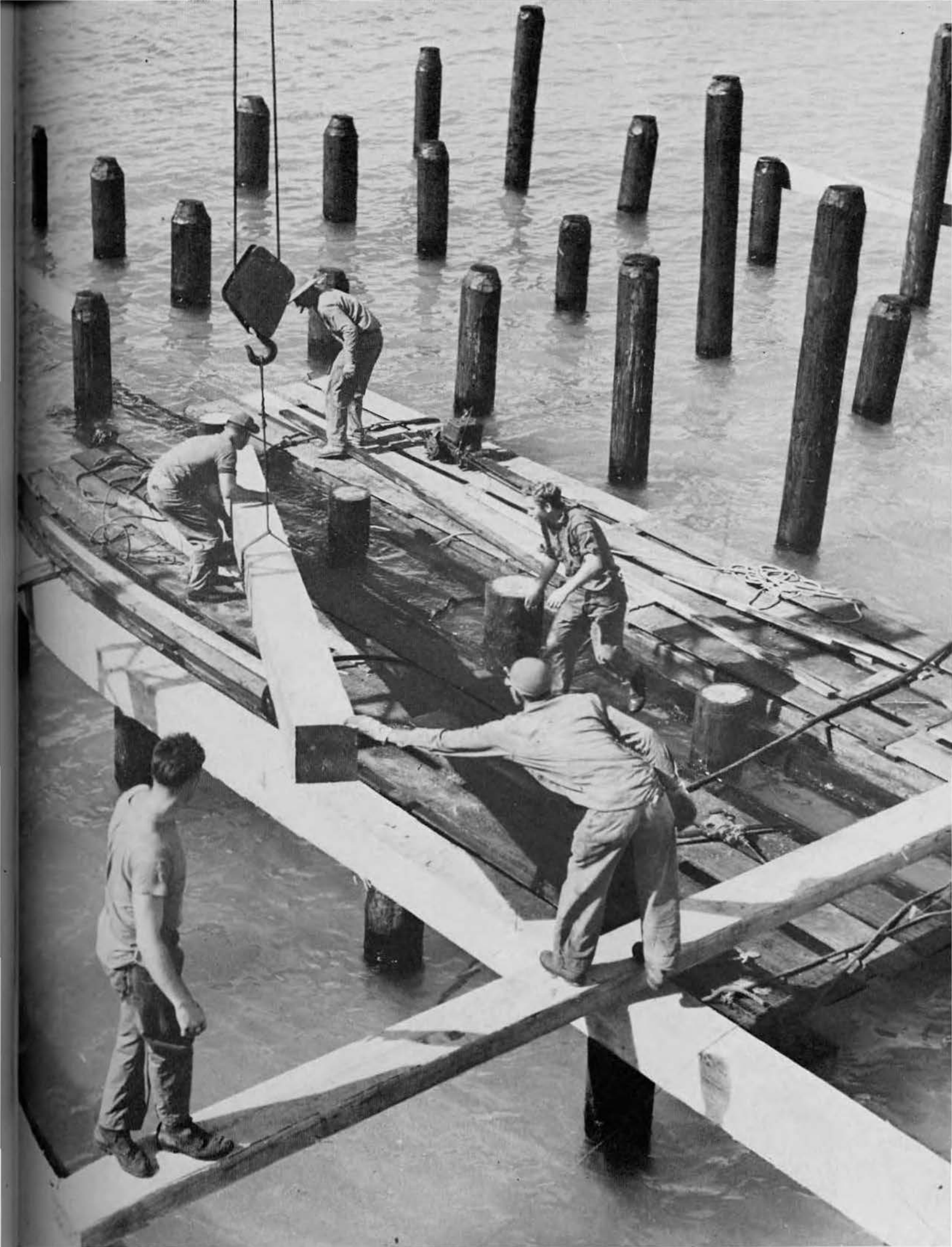
Another waterfront job with a hard-to-meet deadline was this permanent pier to be used in loading war ships.
