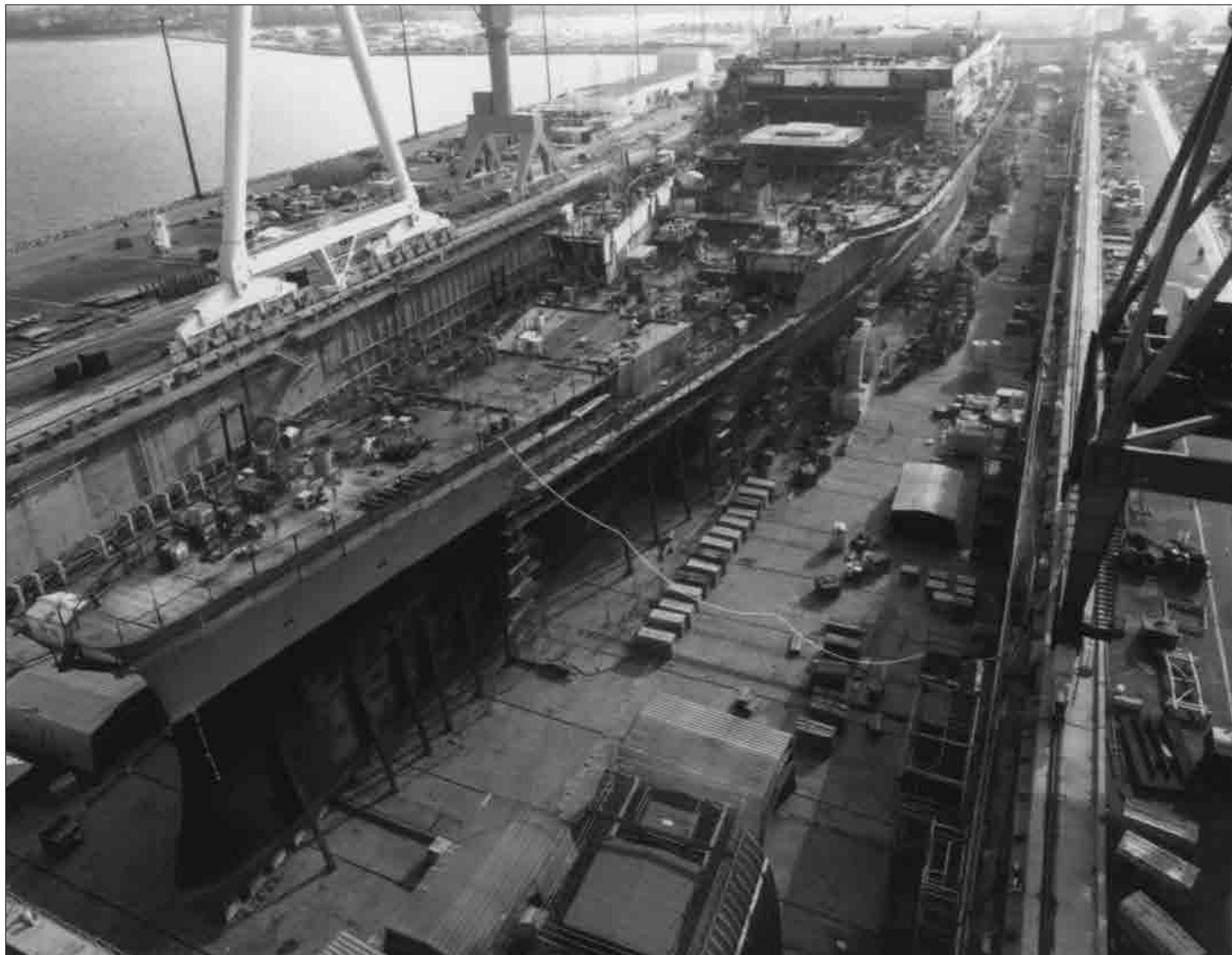
Harry S. Truman (CVN 75), laid down on 29 November 1993, is under construction at Newport News, Va. She was commissioned on 25 July 1998.
