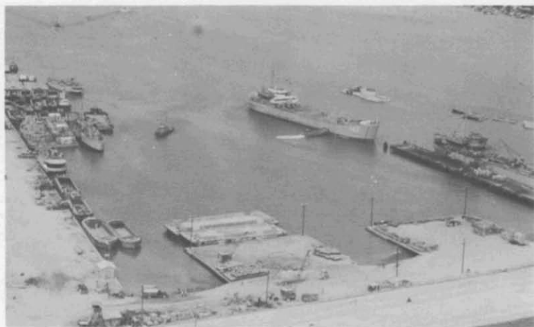
7. Bridge Cargo Facility—Da Nang East. Built by the Seabees. Principal construction features are a 1,700' sheet pile bulkhead, 2 LST ramps, and a 300' wooden pier.
