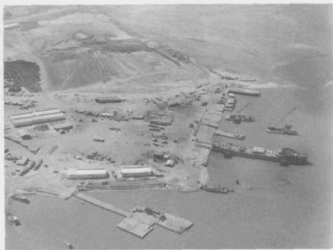
5. Tan My Port Facility. This project included 4 LST ramps, 2 LCU ramps, a barge pier, and a 160,000 SY hardstand.
