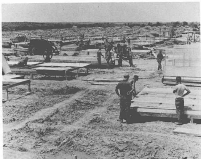
72. "Strongback Huts"—Quang Tri Combat Base. Seabees of NMCB-11 are building hundreds of "Strongback Huts" for a Marine camp. These units were later converted to "SAE Huts" by replacing the tenting with corrugated sheet metal roofing.
