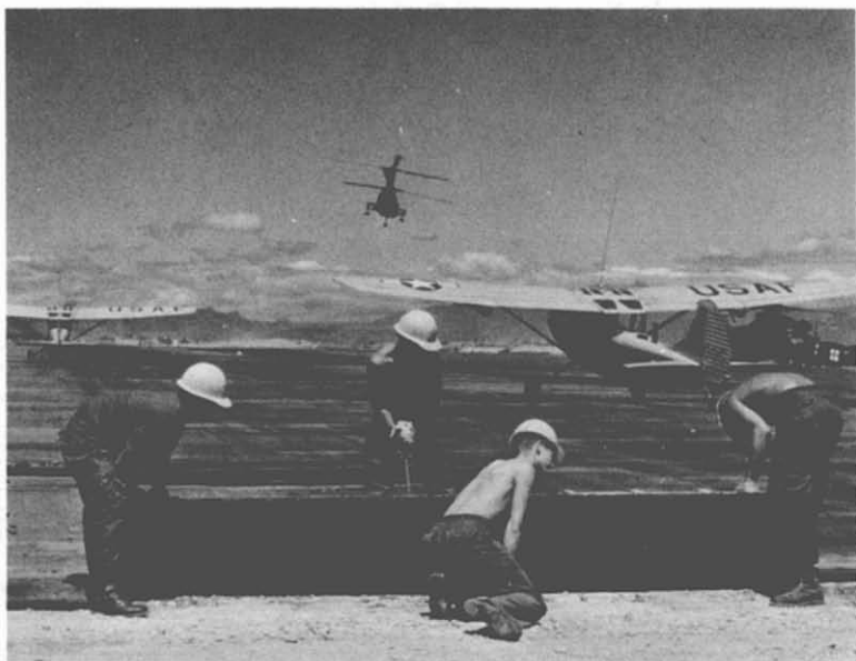
70. AM-2 Runway Repairs—Dong Ha. Seabees of NMCB-11 work on a type AM-2 (aluminum) runway matting that was damaged by enemy fire, as helicopters continue to operate overhead.
