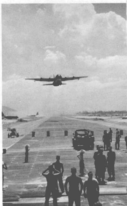
93. Runway Resurfacing—Phu Bai. Seabees of NMCB-133 resurface the runway as a C-130 Hercules aircraft takes off from the completed end of the runway.
