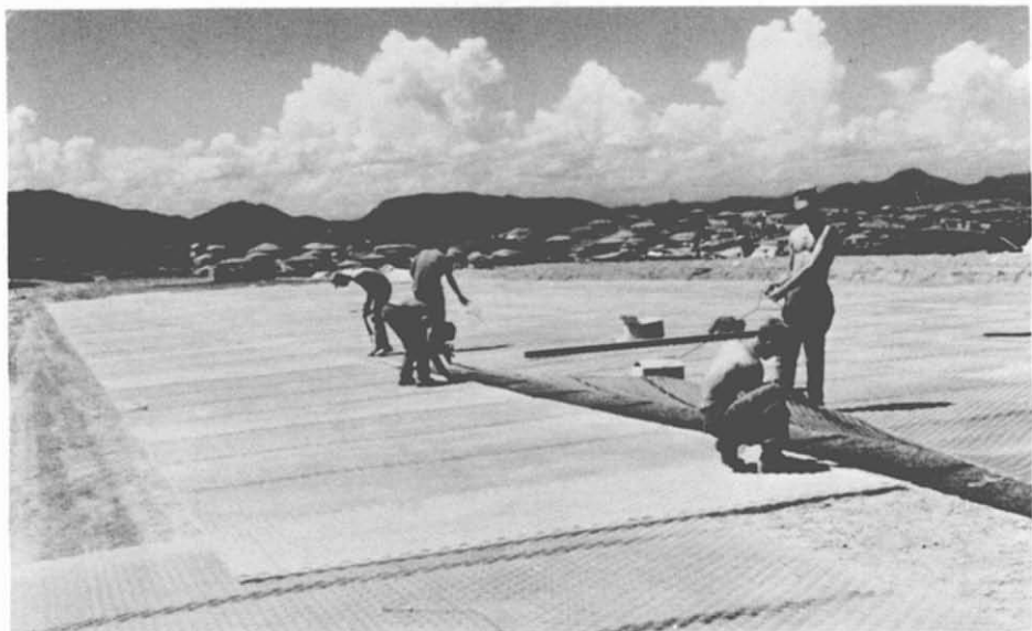
89. MoMat Runway Repairs—Near Hue. A "detail" of Seabees from NMCB-4 positions and splices "MoMat" sheeting on the runway at Camp Evans airfield, located about 20 miles north of Hue.
