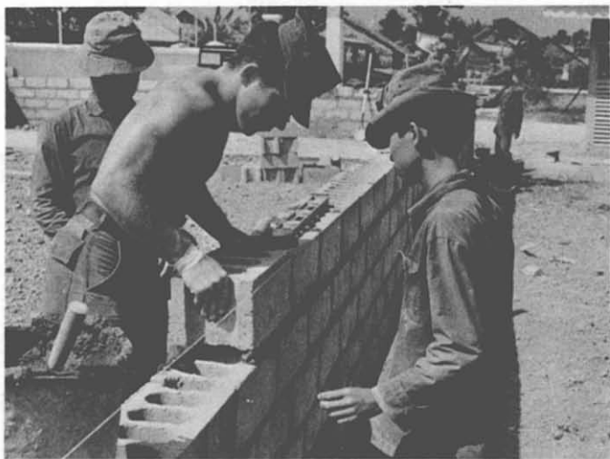
78. Trainee Laying Cement Block—Chau Doc Province. Seabee Tommy Allen of Seabee Team 5803 of NMCB-58 shows Vietnamese trainees the correct way to lay concrete block while building a 10-room nurses' dormitory.
