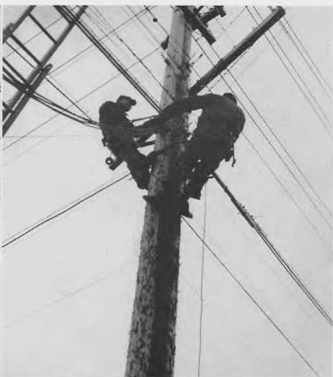
Linemen were at work in all types of weather, keeping communications and power lines in service.
