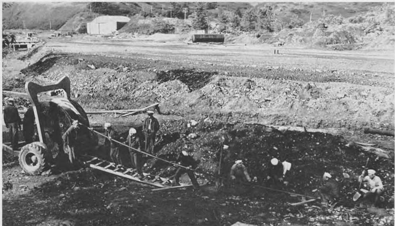
The underground electric department pulling cable. This cable was in fibre conduit, and nine hundred and eighty feet long.
