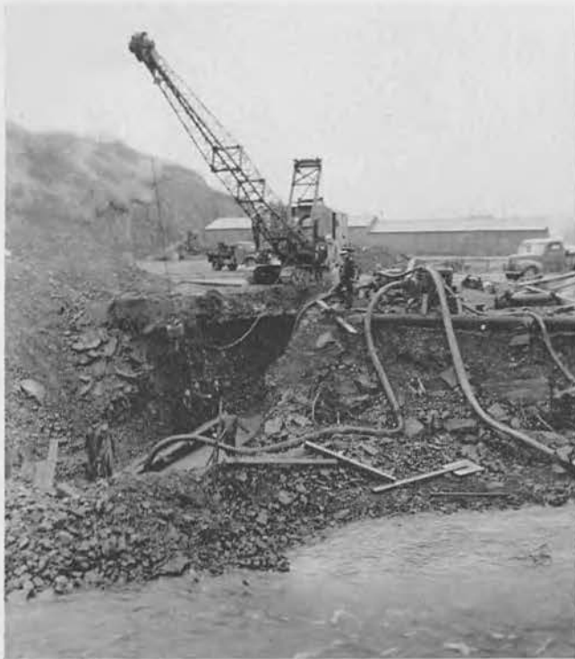
The pipe line was one of our largest projects. Here it is being run under a stream.
