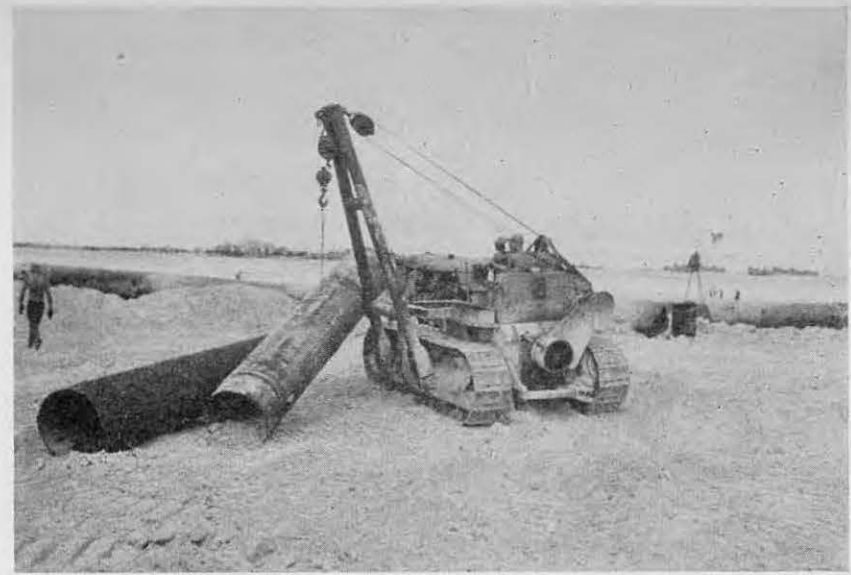
A "cat" with a side "Y" frame moves into place on the fill
