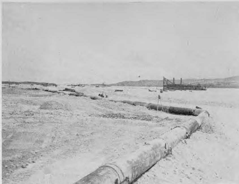
A long pipe line over a fill area, with the YM-19 in the background
