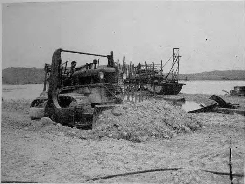
As fast as the dozer smoothed it out, the boys piled supplies on it
