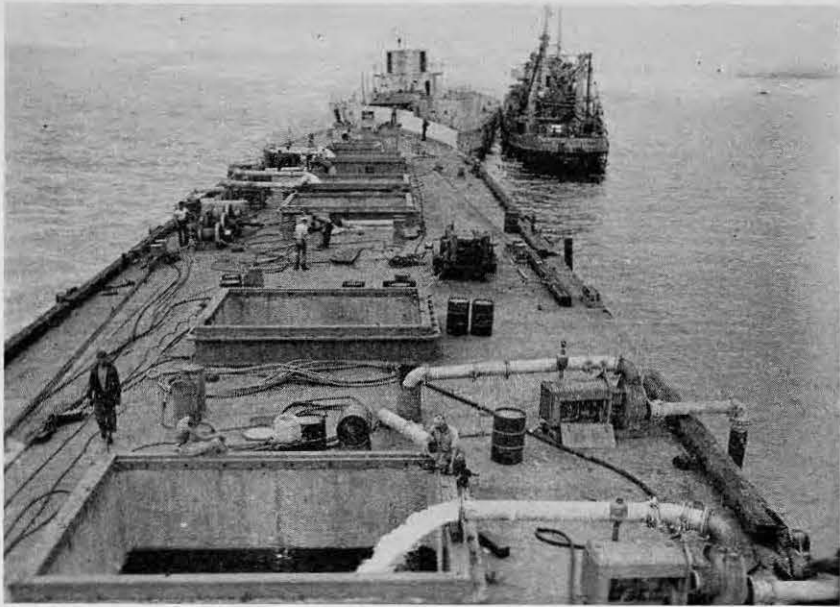
The winches are secured to the deck, and the mooring lines ready, as the concrete is towed to its final resting place
