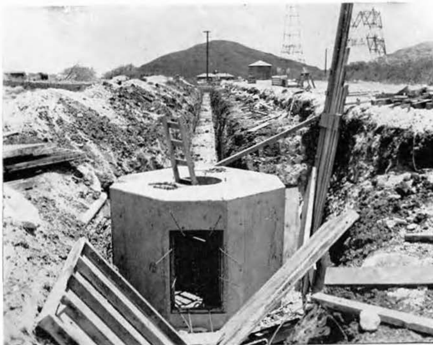
8 miles of underground conduit.
