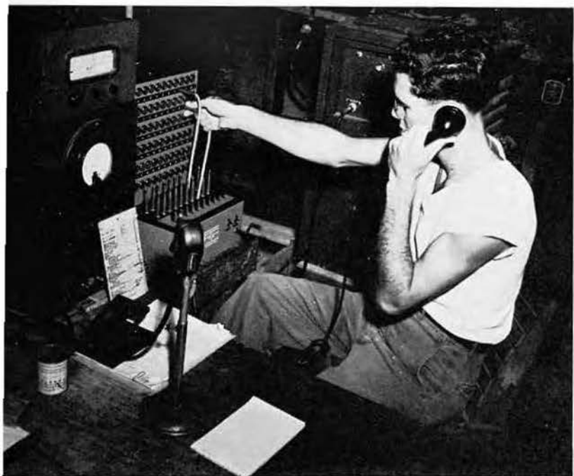
Kenny Goodlad operating switchboard in O.O.D. Office.
