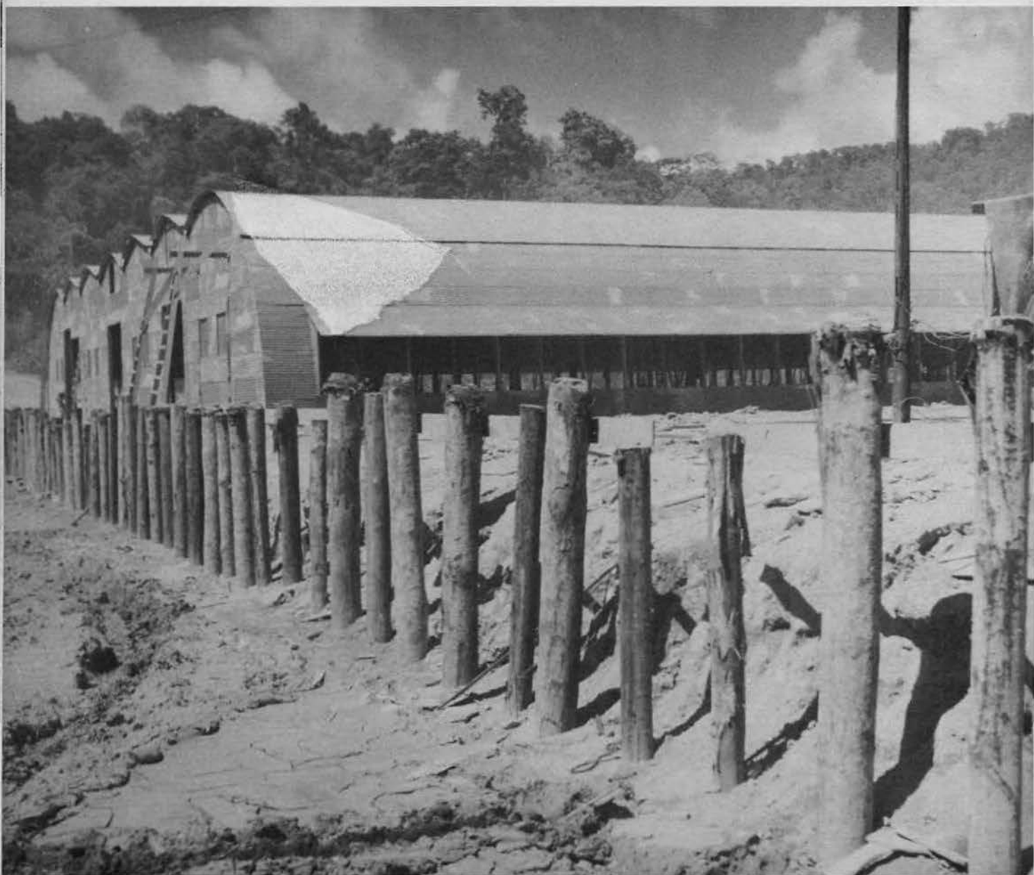
A force of twenty-five Seabees and 150 Filipino workers completed each of the huge structures in an average time of 8 days
