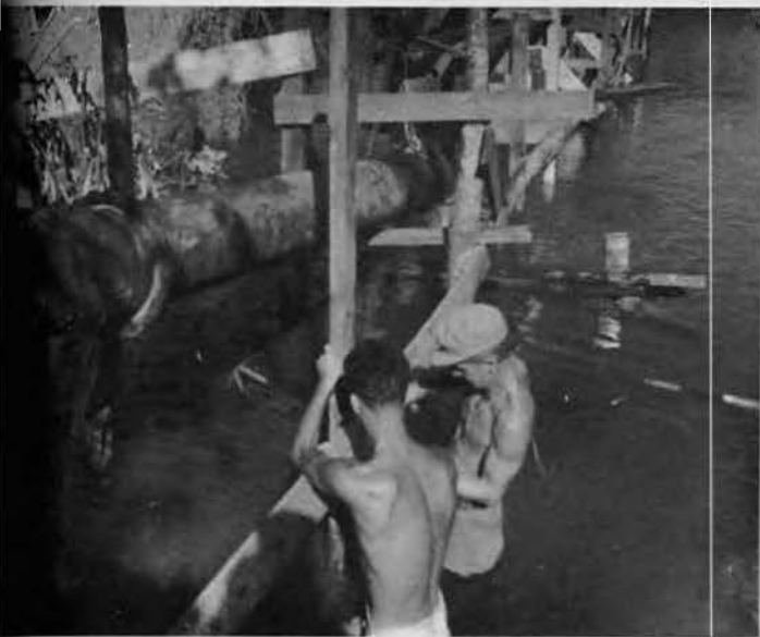
Ship's water supply: pipe line
