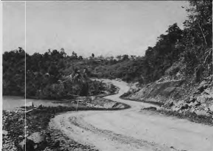
A perfect example of the use of displaced rock and dirt from a steep slope as fill, in the water, to create the road-bed along Hollandia shore line.
