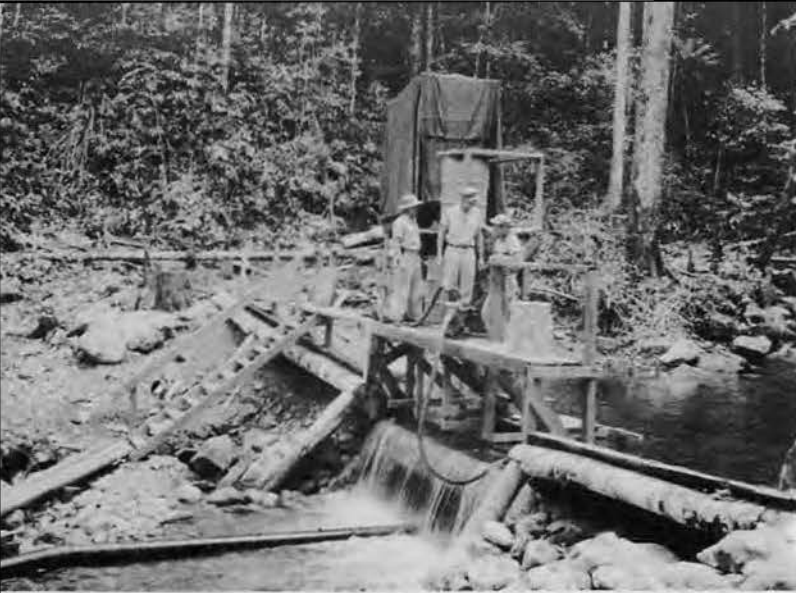
Permanent Naval Base water supply source at Hollandia was at this 113th-constructed dam two miles up Nubai Creek in mountains back of waterfront.
