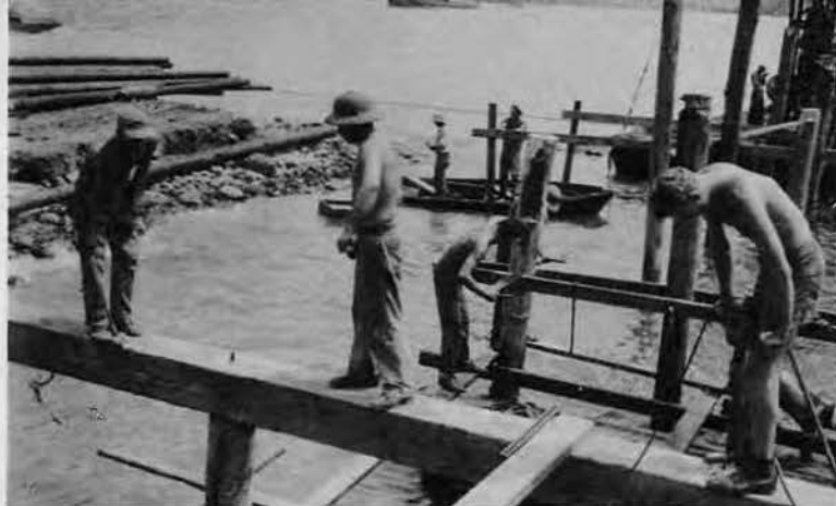
The Hollandia Small Boat Dock slowly takes shape as the Crew follows up the "Joe Magee" floating rig with capping and bracing.
