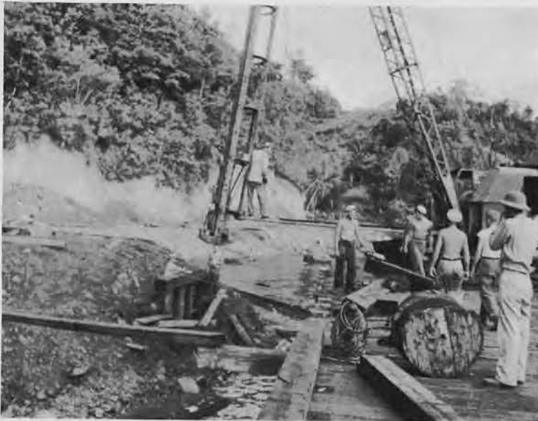
Below: Putting the finishing touches on the rigging of a shovel to serve as pile driver.
