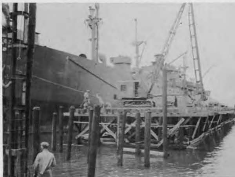
Land pile driver stands by on Dock No. 1 as Crew sets piling that has been spliced by the men in upper photo.
