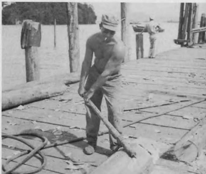
Strong arm preparations for driving the final pile at the Pie Beach Small Boat Dock.
