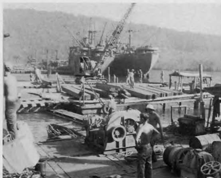
Unloading timbers from a pontoon barge for Small Boat Dock construction. The photo, taken from the floating clamshell rig, shows part of the channel dredging equipment mounted on pontoons in the foreground.
