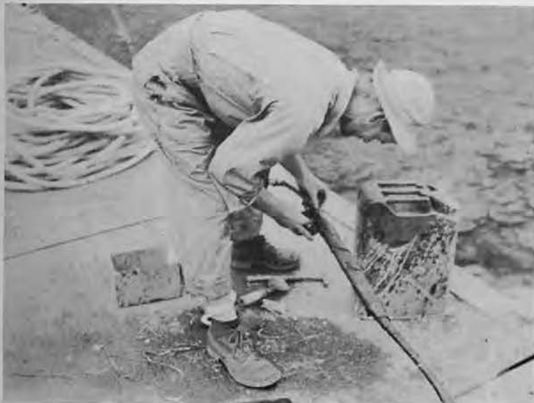
Making one of the five splices used on the 17,000 feet of submarine cable laid from NAB to Imbi Point. Cable was laid in 143 feet of water.
