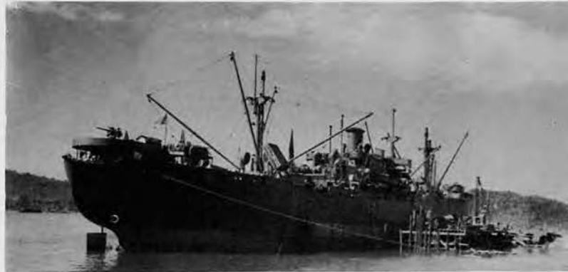
Sixteen days after the driving of the first pile for Dock No. 1 this picture was taken as a Liberty Ship discharged cargo onto a portion of the Dock.
