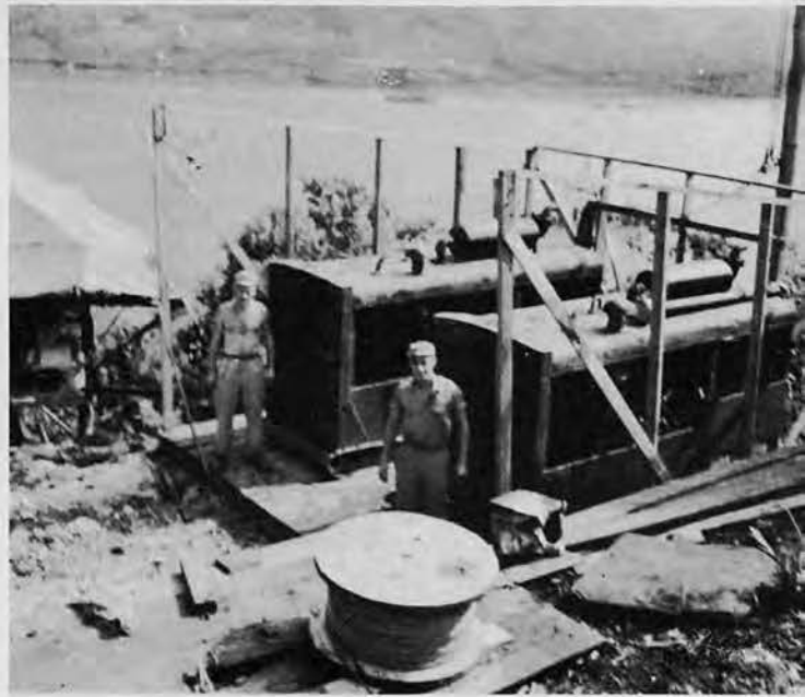
Partially completed Generator Station at top of Signal Hill. Generators are already in operation, before building is completed.
