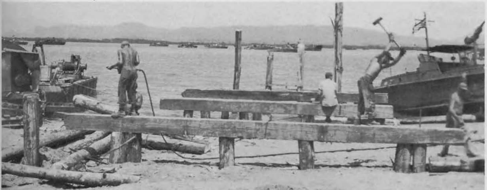
The beginning of construction on finger piers for Motor Torpedo Base at Mindoro. PT boats may be seen anchored in the bay.
