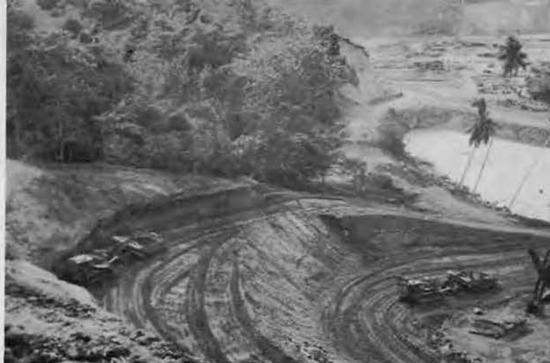
Carryalls make wide loop to gather dirt from side-hill borrow pit for fill at right center.
