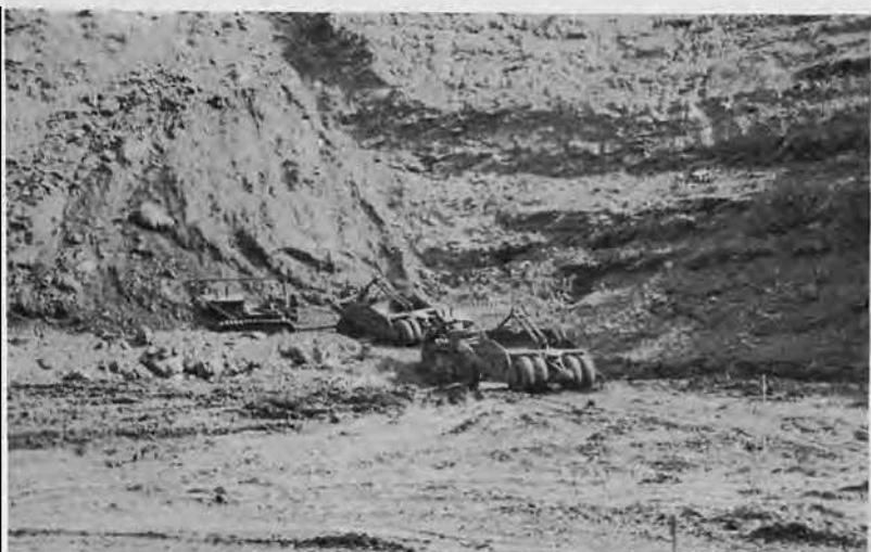
In the construction of the Sorting Docks near the LST watering point, extensive fills were made from coral and rock pits. Here carryalls are operating in a borrow pit near Graveyard Cove.
