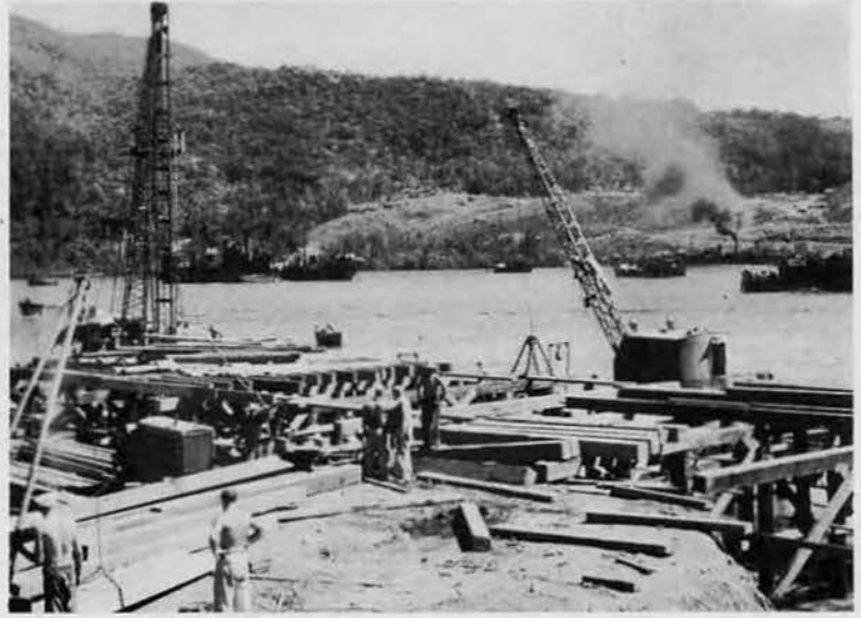
The A-frame in the foreground deposits timbers for deck. Clamshell at right center dredges the bottom to Liberty Ship depth.
