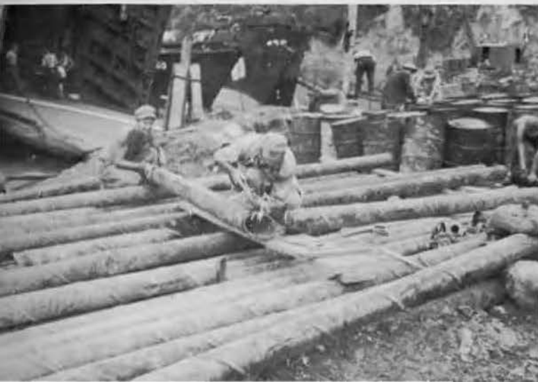
Welders prepare joints for Base Water Supply System while landing craft take on water in background.
