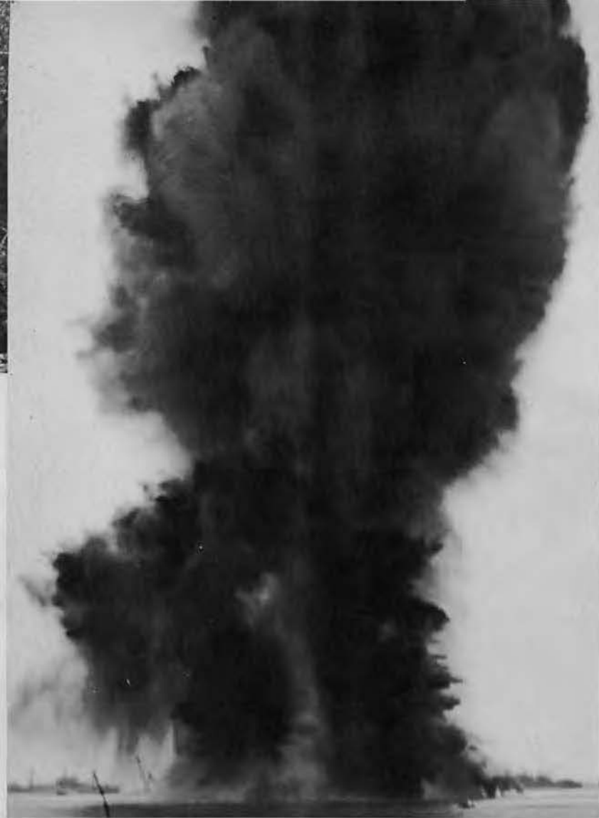
Above: "The sound and the fury" cut loose as channel is blasted for Officers' Small Boat Dock. Below: Blasting Crew lays hose filled with TNT prior to blasting of channel.
