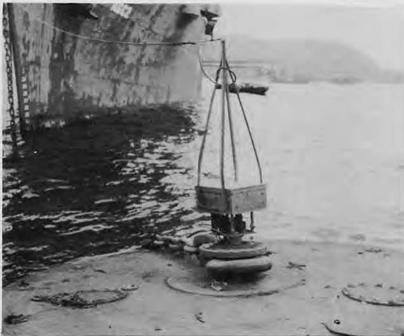
Telephone terminal box atop cruiser mooring buoy, with cruiser "plugged in" for telephonic communication.
