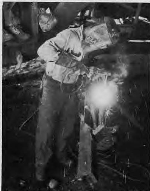
The be-hooded "Penny Flash" strikes an arc while working on a repair for one of the motor graders.
