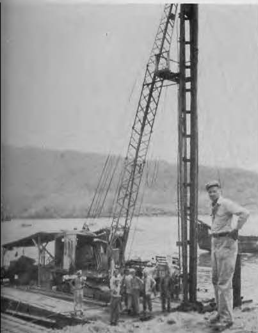
The "Joe Magee" floating pile driver, drives first piling at start of construction of Navy Dock No. 2.
