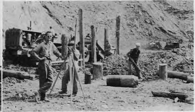
Preliminary work on retaining wall for sorting docks at Graveyard Cove is lined up by Surveyors.
