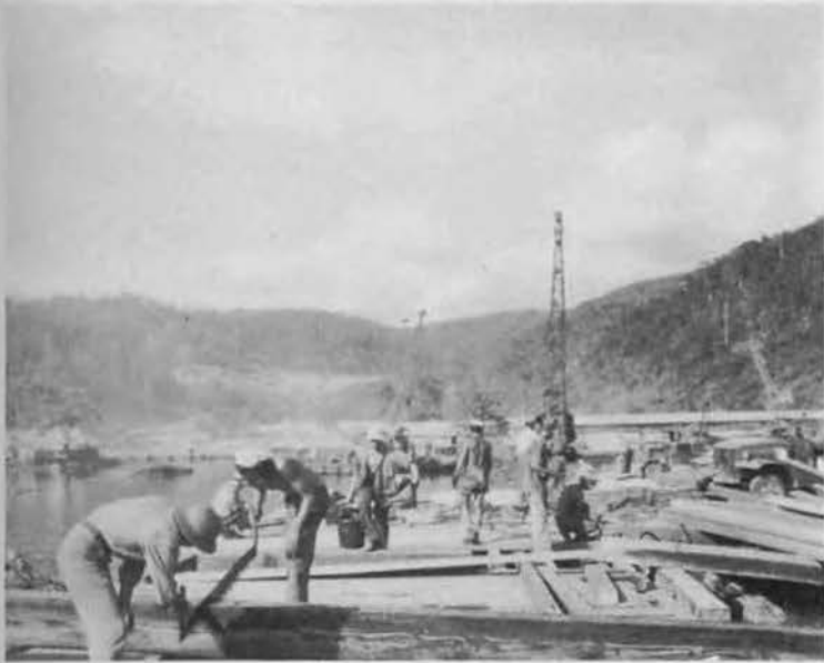
Close-up of dock construction. Note the ease with which the two men in foreground operate the "manpower" crosscut saw.
