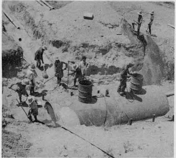
5000 GALLON TANK. Installing one of the two 5000 gallon septic tanks incorporated in the sewage disposal system for the camp by CBMU 606. Frank Mannella is the welder shown in the picture.
