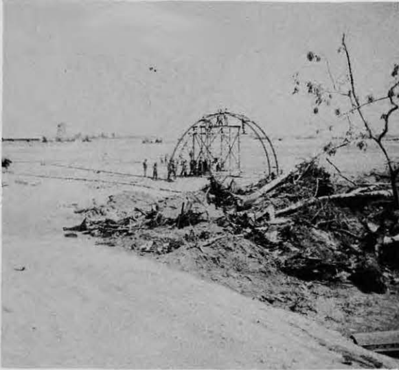
STEEL HUTS. Progress photograph showing start of the first 40 feet by 100 feet Stran Steel Huts to be used for aviation facilities at the Clark Field air strip.
