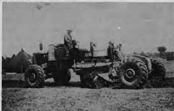
MAKING ROADS FROM RICE PADDIES AT THE MANGALDAN CAMP. Upon arrival at the Mangaldan camp site the road building division of CBMU 606 hastily built adequate roads throughout the camp.
