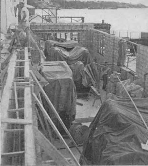
Battery Charging House
