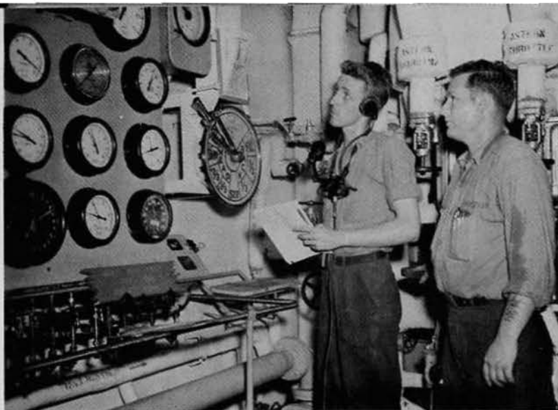
ENGINE ROOM GAUGE CHECK
